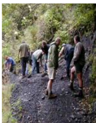
Help off-road recreation by doing the right thing. There are lots of ways to get involved and you'll have fun doing it. Photo: 4WD club repairing a 4WD track, DOC
